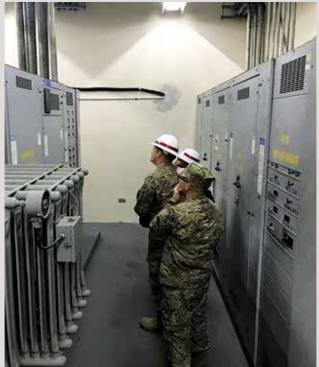
Supporting Puerto Rico after Hurricane Maria, 1st Sgt. Villalona provides language support in maintenance checks of existing power.
